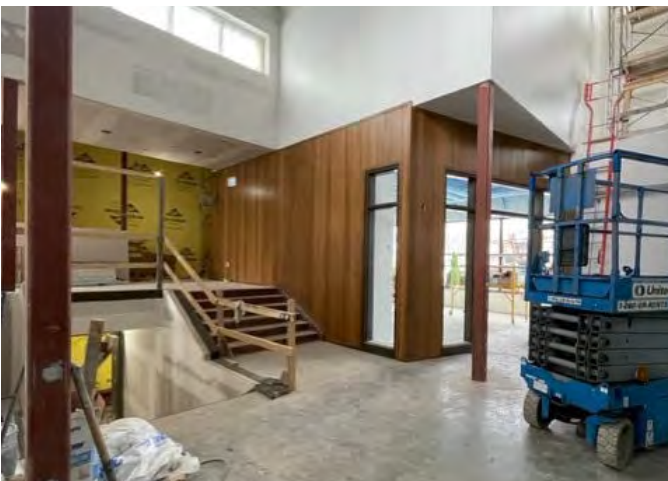
The wood paneled room will be the Creative Classroom, which is right next to the stairs leading to the Carnegie building side of the library
