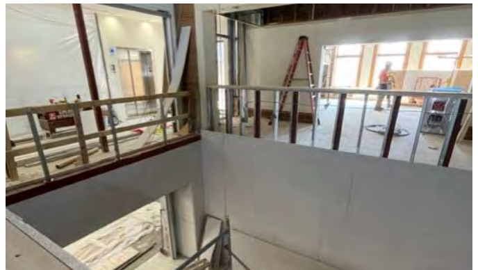
Looking south toward the East Reading Room, there is now an opening to the lower level behind what used to be the main service desk.
