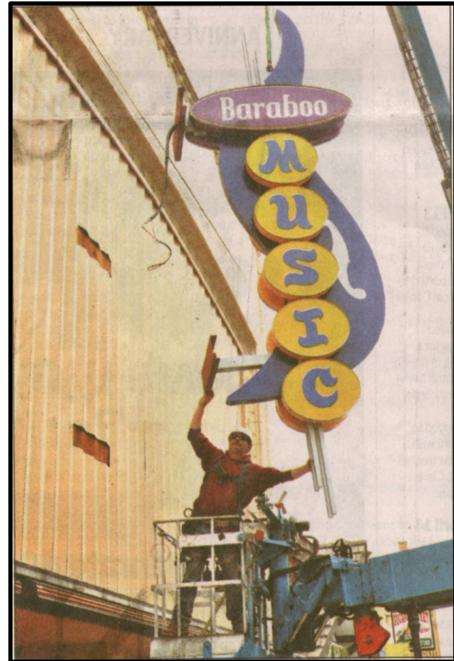
In April of 2012, the La Crosse Sign Co. of Onalaska installs a new sign at 129-133 Third Street
